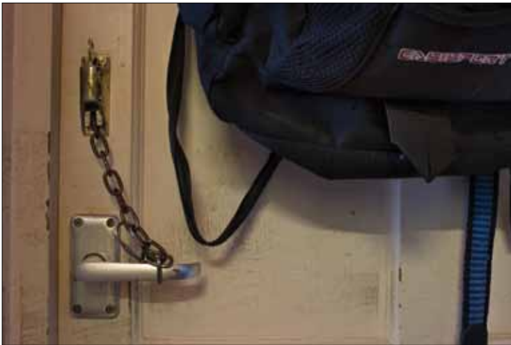
Figure 3 The entry doors to the flats are flimsy, and a resident has devised this safety contraption.
