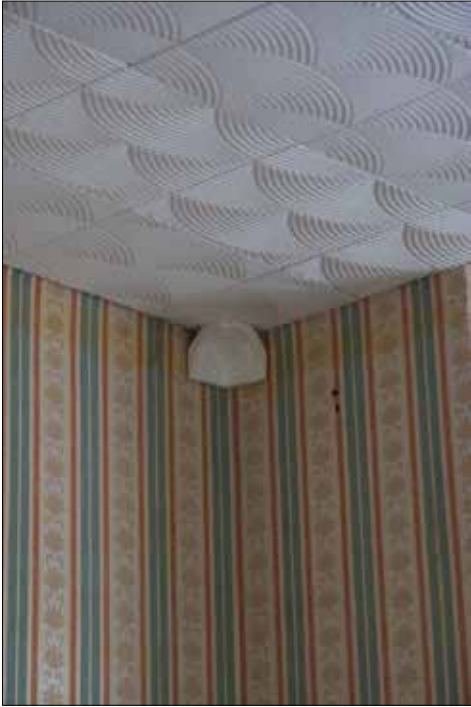
Figure 15 Plastic ceiling tiles. Empty flat.
