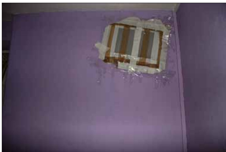
Figure 21 Nearly every flat we photographed had taped up the air vents, as the flats are drafty and very cold in Winter.
